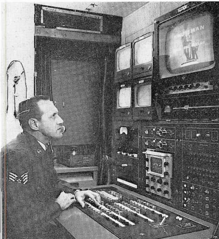
FIG. 11. TV switching system Type TS-40 selects program source requested in any of the conference rooms or offices. System permits special effects to be inserted.
